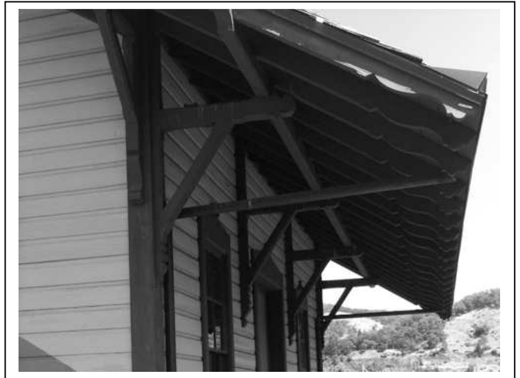
O&C bracket design seen in the Dillard depot (right) was retained at the remodeled Gold Hill Depot (below). [Larry Mullaly photos. below, SOHS photo Box 639F5]
