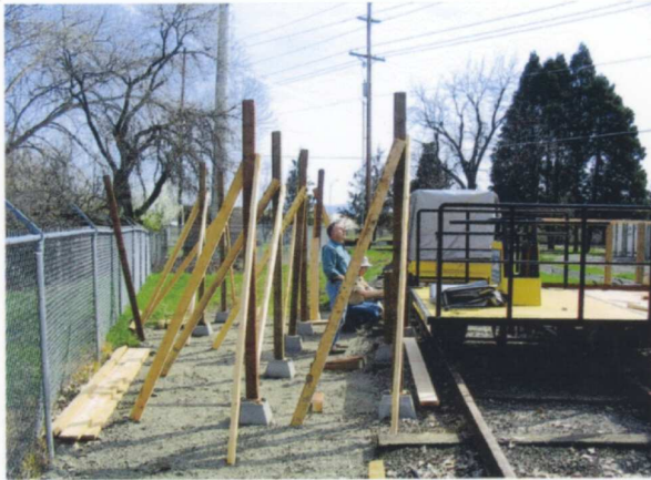
(LEFT) Is Bruce McGarvey looking for rain or divine intervention? Despite the bad weather in March, the work on the new loading platform for our handcar and motorcars picked up steam. Here Bruce is checking the level for each post so that everything added afterward will be perfect.— Rick Aubin photo
