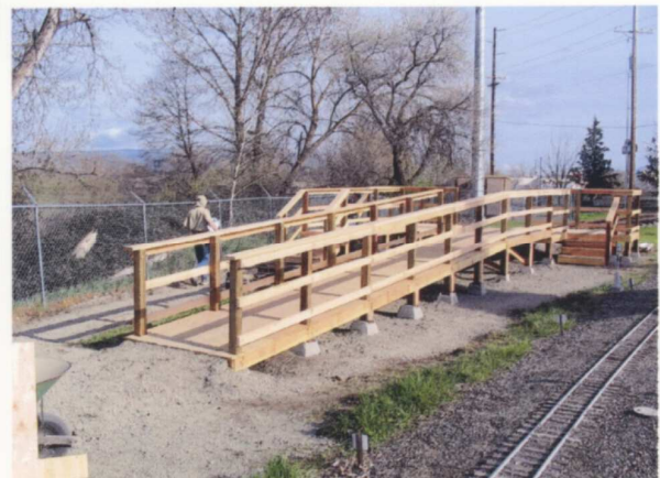
(RIGHT) A little closer view shows how well project coordinator Brian Fraiser planned this ramp. He built this ramp as part of his Eagle Scout requirement for community service. New plastic handrails are now in place since this photo was taken. — Rick Aubin photo
