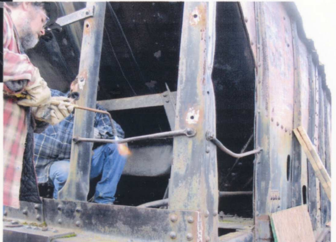
(RIGHT) From this angle you can see how severely bent some of the rungs are. Those that can be straightened are done in place, while those too crooked are cut off and new rungs will be fabricated instead. — Rick Aubin photo
