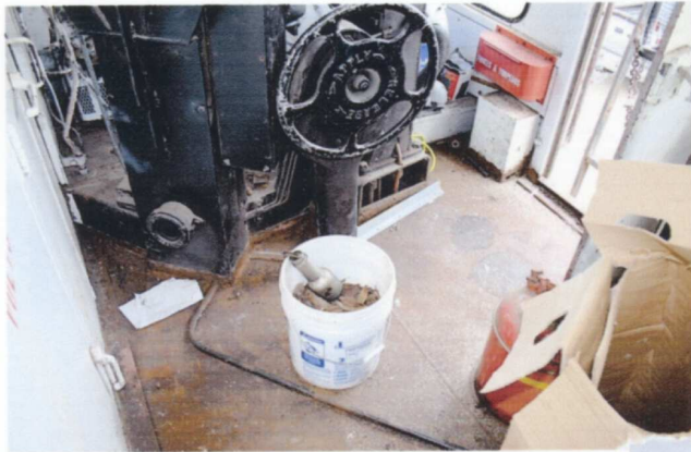
(LEFT) This is the floor inside the cab of Medco No. 8 after the wood floor was removed. The old wood was likely the original floor installed by Baldwin-Lima-Hamilton back in 1952. A new floor will be installed after painting the locomotive. — Tony Johnson photo
